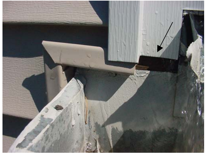
Water goes right behind this new vinyl siding at the end of the gutter. This problem is very common.
